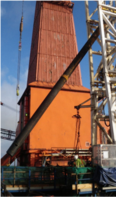
The Mastiff RIS performed casing and conductor recovery on 23 platform wells prior to removal of the topside platform module.
